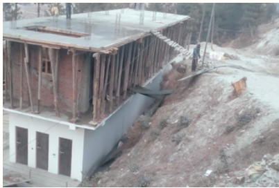
Construction in Mugu, Nepal has been completed thanks to Dr. Margreet Hogeweg
